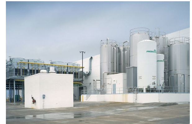
Image 3.2 Exterior equipment on a cold facility.
